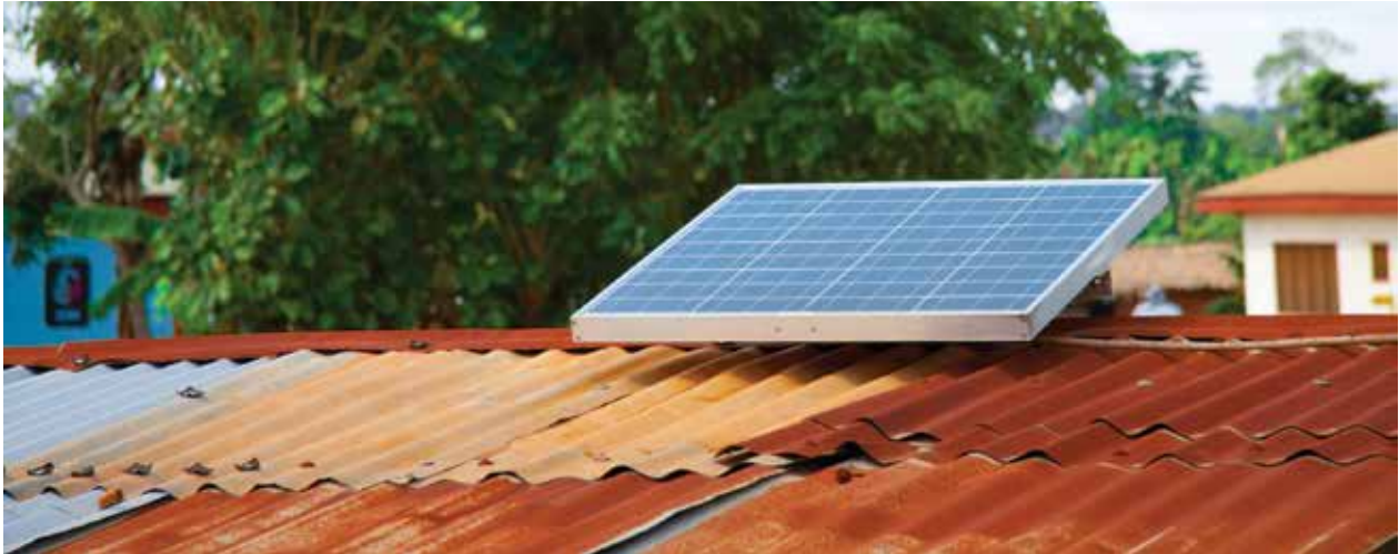
Rooftop solar panel in Ghana.
